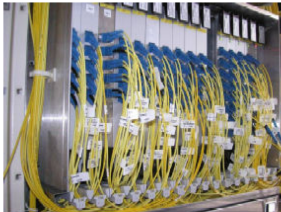
Figure 14 – Example of Several Installed Network Units
